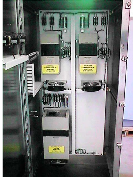
Figure 6. CVT enclosure internal components i.e. CVTs, fans, fuses, and termination blocks.
